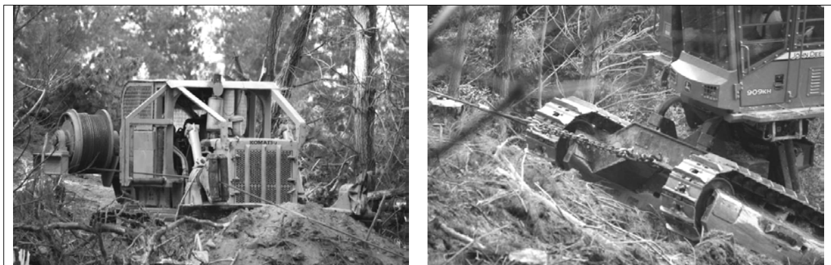
Figure 2. Purpose-built self-levelling harvester (right) being cable-assisted by the winch mounted on the dozer (left).
